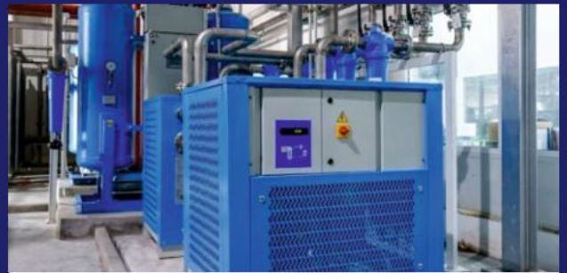
Compressor and plant systems
